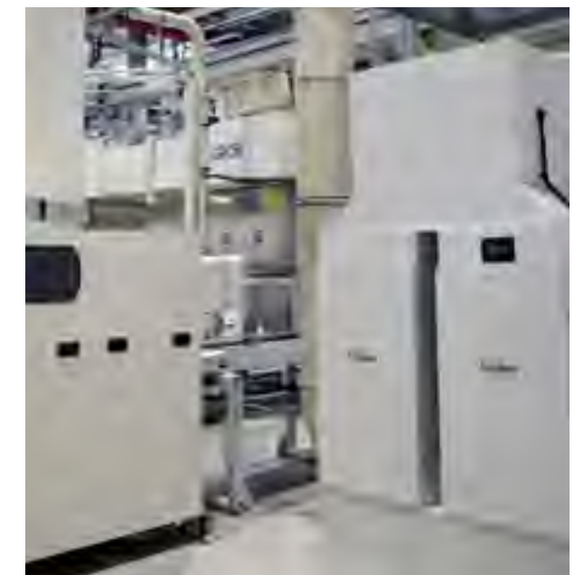
Absolent installation at MAN, Germany. Solution: A-mist80TF (one filter unit for each machine)
