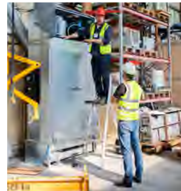
Absolent installation at Pyrotek, Sweden. Solution: AD051 (the first ever AD unit installed)
